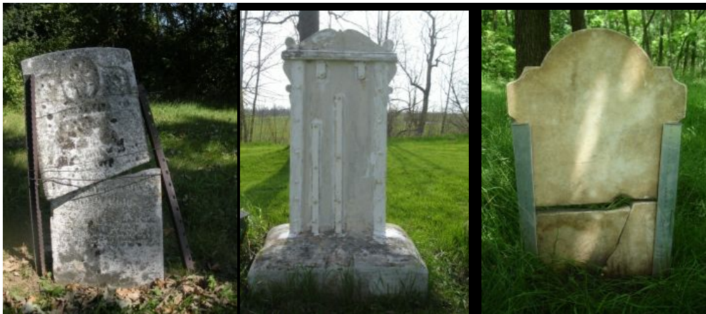
Figure 3.17. Repair work at the Clark, Lymburner, and Swayze Family Cemeteries, showing the extensive use of metal, most extreme in the centre image where struts have been bolted into the marble and painted.
